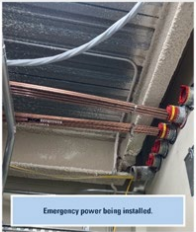
A small portion of the many many cables and wires being installed throughout the hospital.
